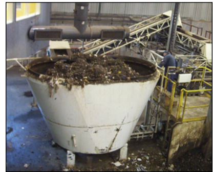
Photo 5-2: Vertical mixer used at a composting facility © Scott Gamble
