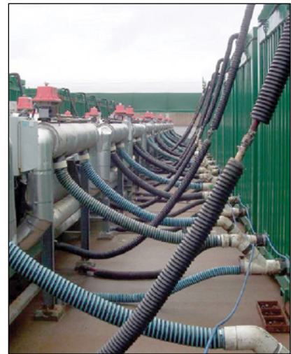
Photo 5-22: Each static container is attached to a central air system using flexible hoses © CH2M HILL
