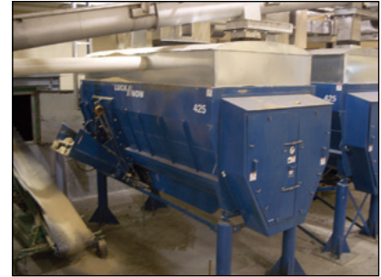
Photo 11-5: Horizontal auger mixer © CH2M HILL
