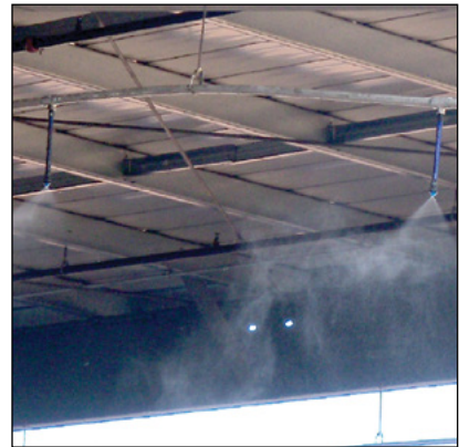
Photo 15-2: Roof-mounted and directional misting systems installed inside buildings and around equipment are effective at controlling dust levels © CH2M HILL
