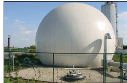
Photo 4-1: Biogas storage tank © Organic Waste Systems Inc.
