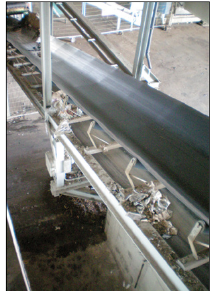
Photo 11-15: Conveyor belts provide efficiencies in moving large quantities of materials within a processing facility © CH2M HILL
