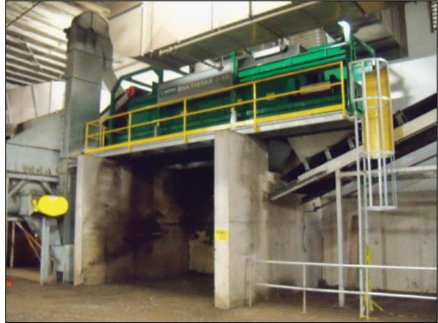
Photo 9-5: Designers should provide appropriate ladders and catwalks so equipment can be easily accessed for inspections and maintenance © CH2M HILL
