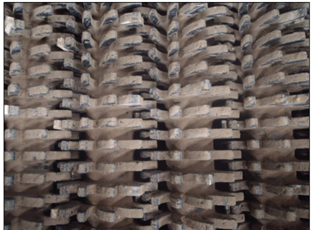
Photo 11-8: Top view of a series of shafts with rubber stars in a star screen (material flow is from left to right across the deck) © CH2M HILL
