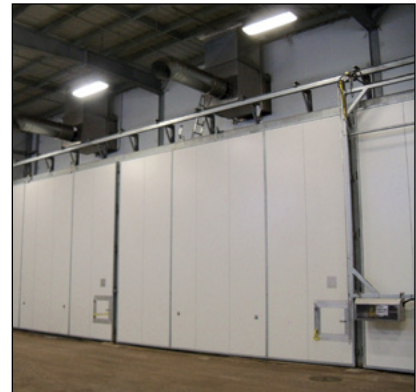
Photo 5-18: Closeup of tunnel door system © CH2M HILL
