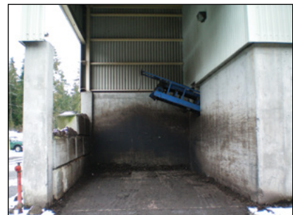
Photo 9-4: A temporary storage area can decouple systems in the facility and provide operators with some flexibility to schedule daily tasks © CH2M HILL
