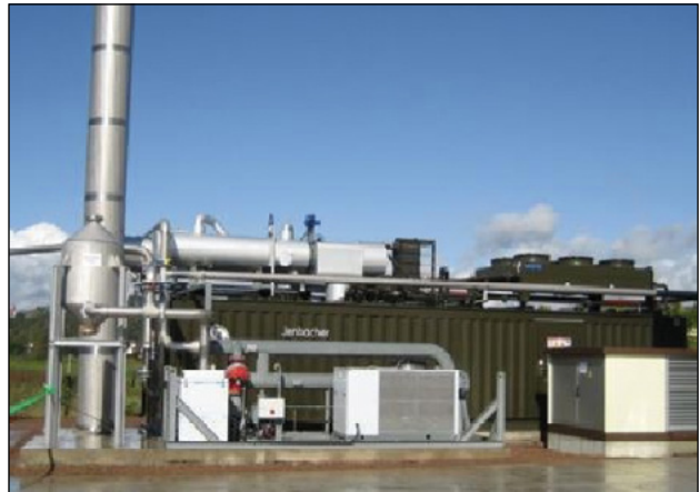
Photo 7-1: Package CHP system © CH2M HILL
