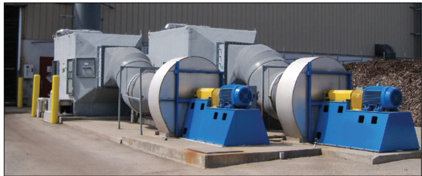
Photo 14-5: Atomized mist scrubber © CH2M HILL
