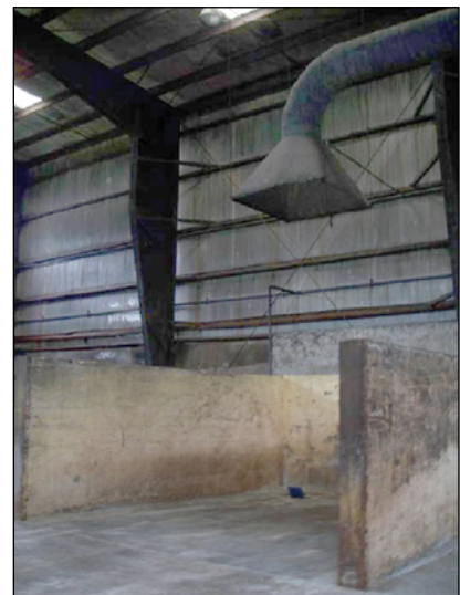
Photo 9-6: Source-capture systems should be used to capture odours before they disperse within the building © CH2M HILL
