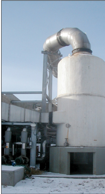
Photo 14-4: Packed-bed tower wet scrubber at composting facility © CH2M HILL
