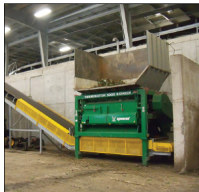
Photo 11-13: Shredding units are common in SSO processing facilities © CH2M HILL
