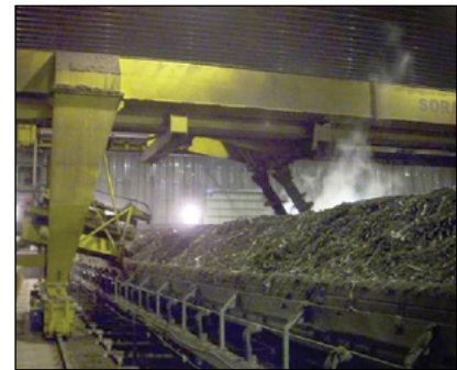
Photo 5-27: Bridge crane and suspended auger turning mechanism viewed from discharge side of bay © Scott Gamble
